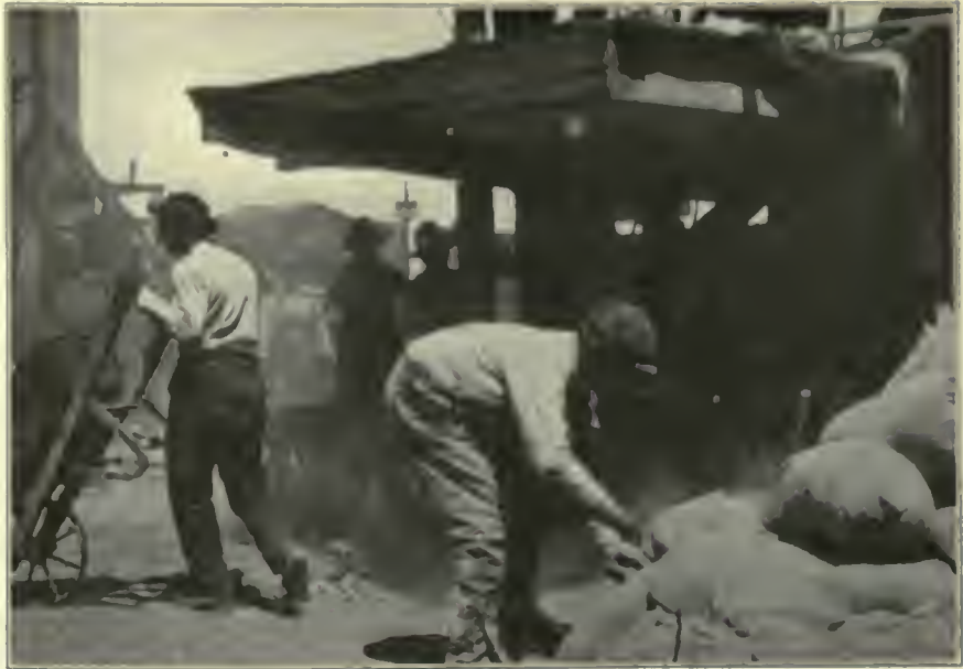
FIG. 47. BUILDING OPERATIONS, A SOURCE OF DUST. The handling of cement scatters fine dust, and the removal of crushed stone and sand from piles in the street leaves the latter but "shovel clean." The residue becomes dry and is blown away by the wind.
